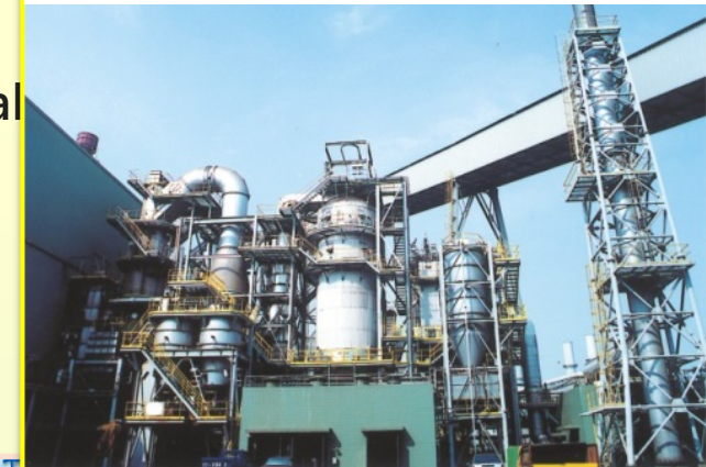
Air Pollution Control System Plant
